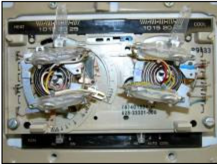
Prohibited: Mercury switches in a thermostat
