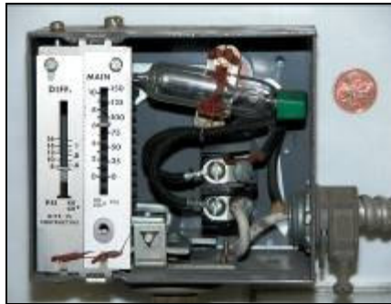
Prohibited: Mercury in pressure and temperature gauges
