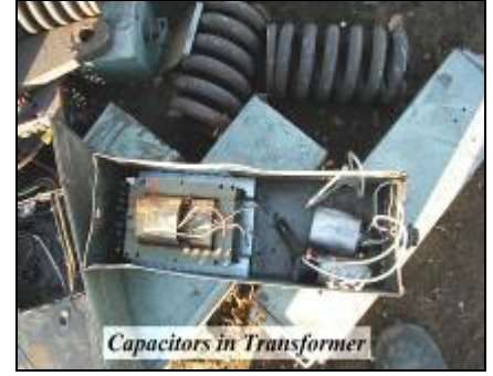
Prohibited: Capacitors in transformers
