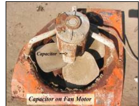
Prohibited: Capacitor on fan motor
