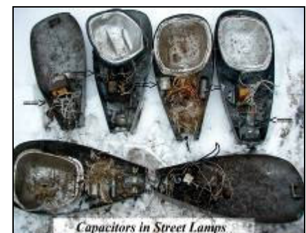
Prohibited: Capacitor in street lamps
