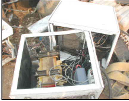
Prohibited: Capacitors in transformers
