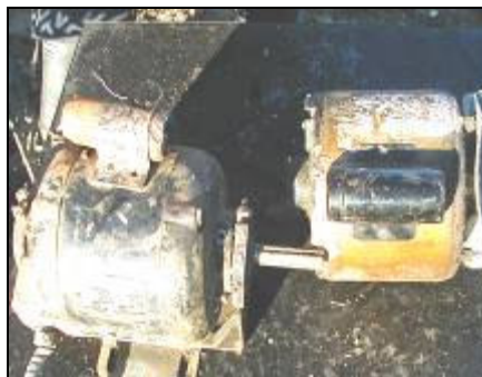
Prohibited: Capacitor in AC motors
