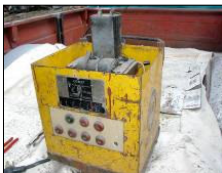
Prohibited: Capacitor in welder
