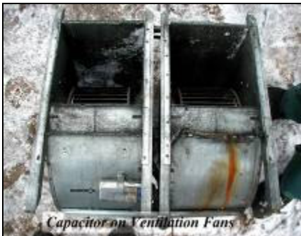
Prohibited: Capacitor on ventilation fan motor
