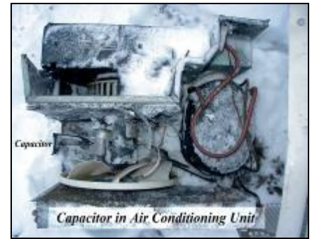
Prohibited: Capacitor in air conditioning unit
